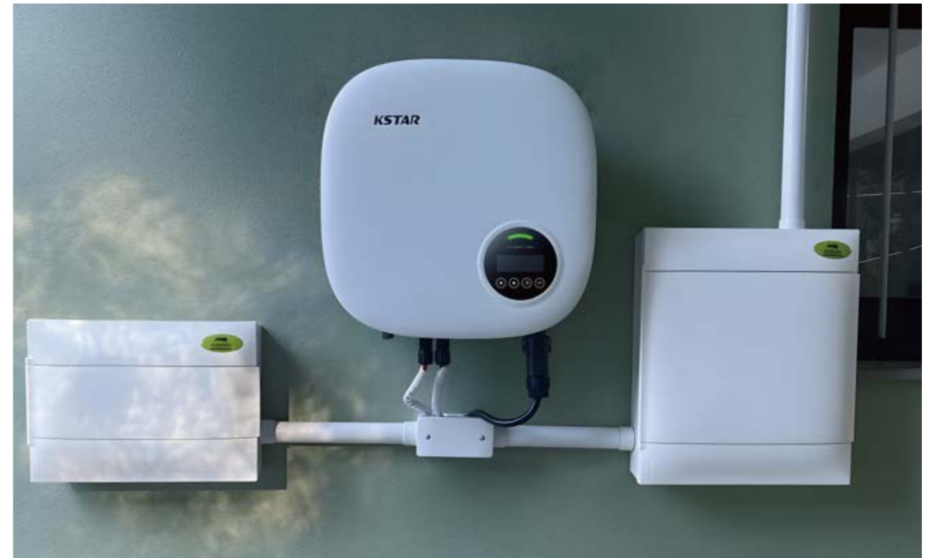
11 Residential Solar Project in Brazil
