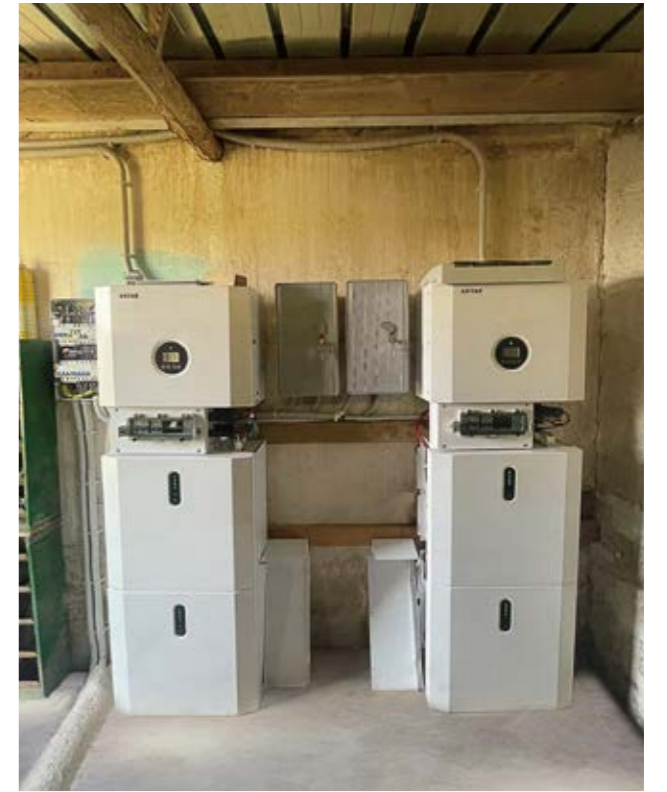
09 Residential ESS Project in Italy
