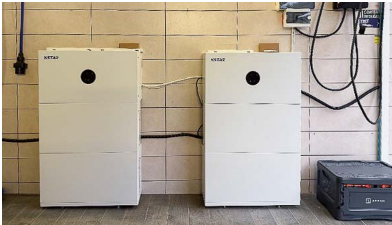
05 Residential ESS Project in Ukraine
