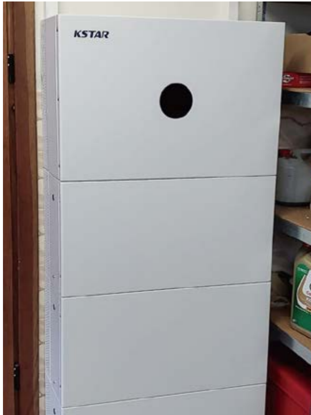
01 Residential ESS Project in Lithuania
