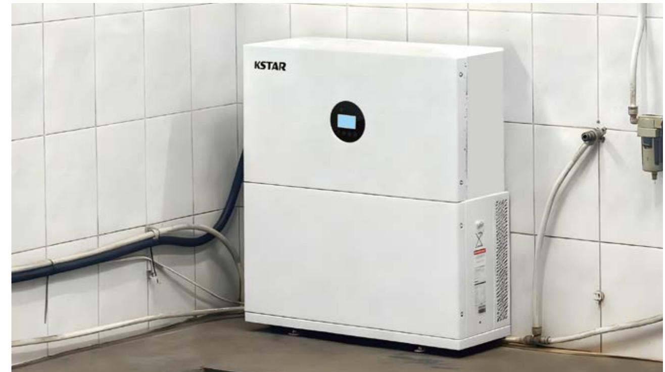
06 Residential ESS Project in Ukraine
