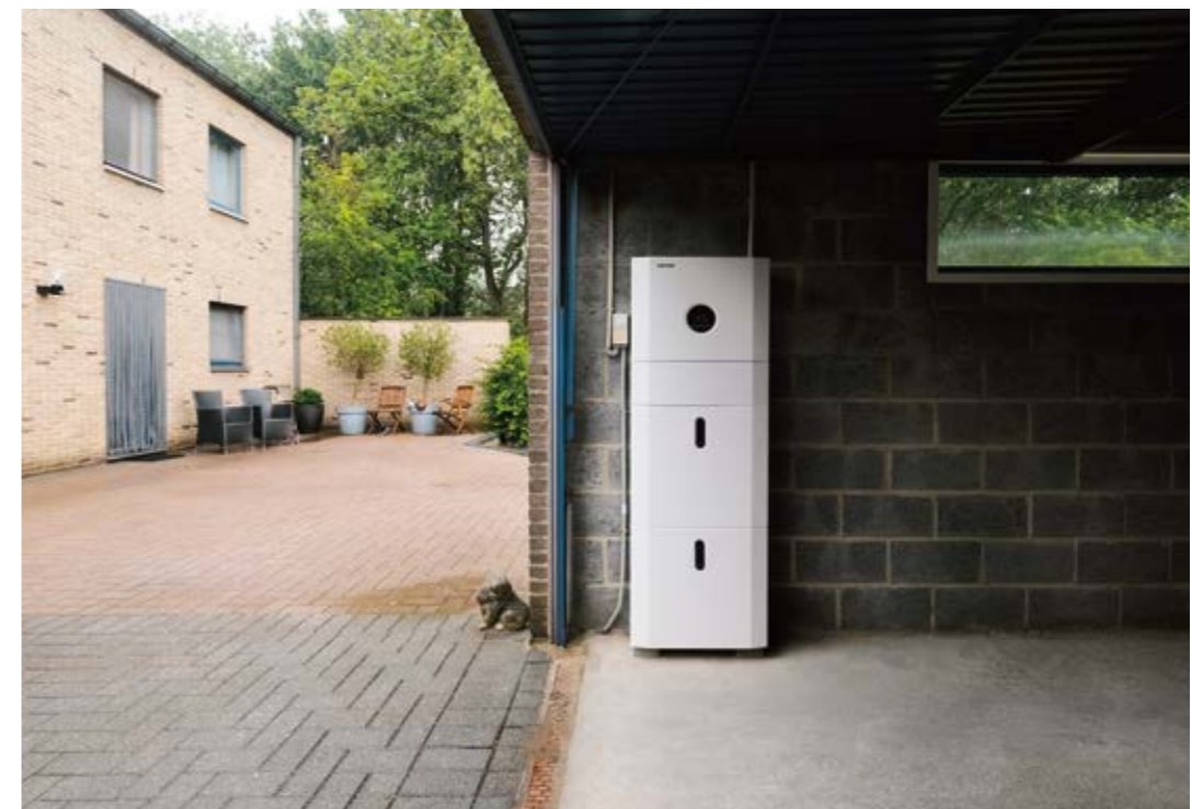
15 Residential ESS Project in Belgium
