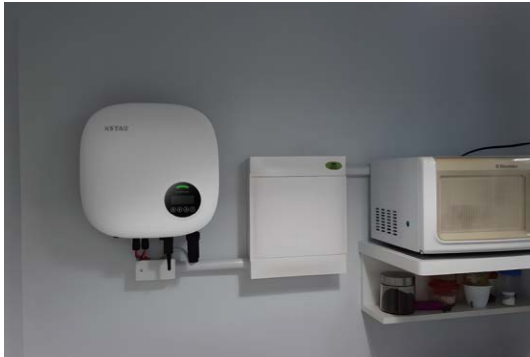
14 Residential Solar Project in Brazil
