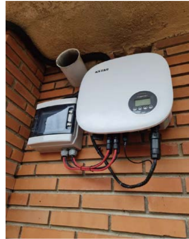
08 Residential Solar Project in Brazil
