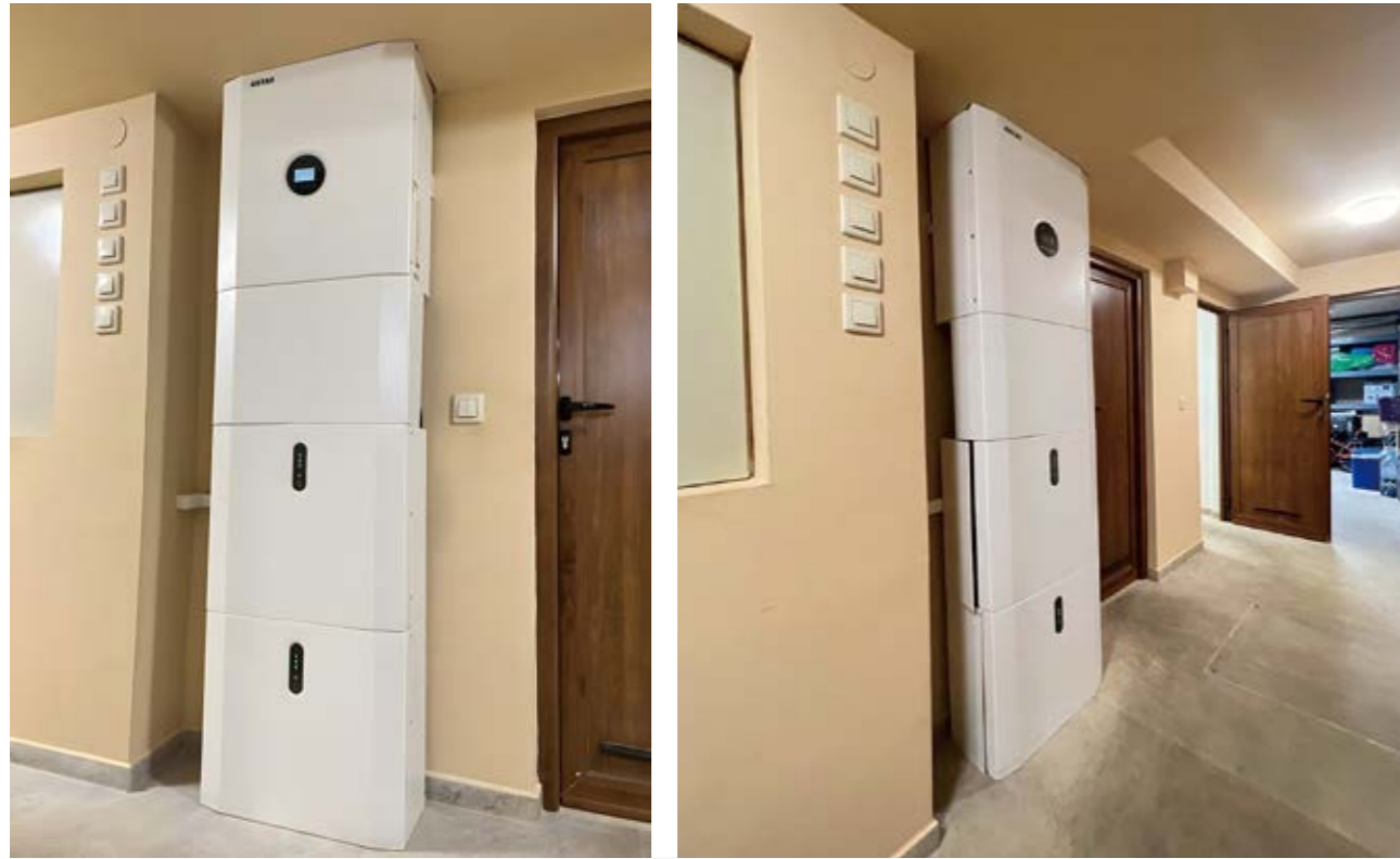
07 Residential ESS Project in Bulgaria
