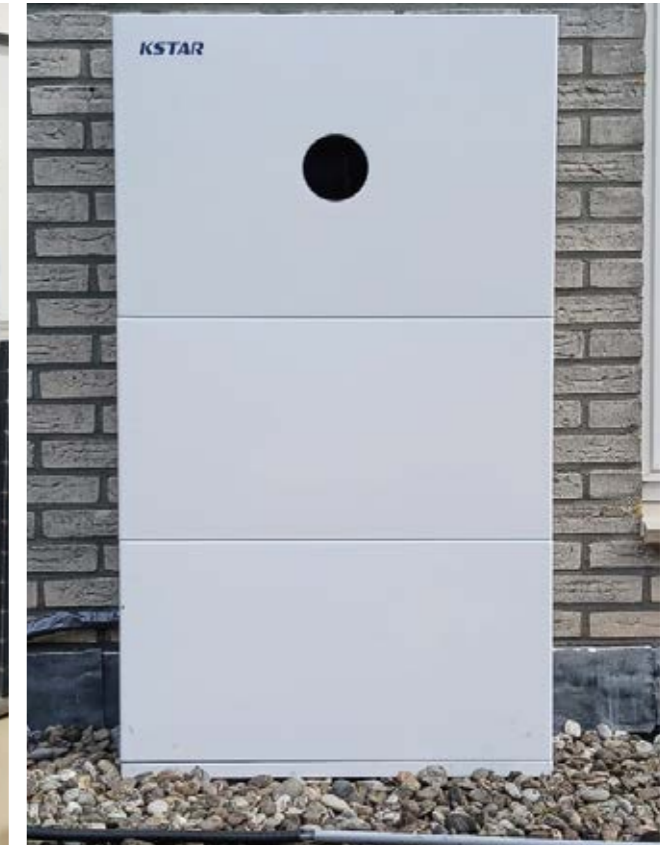
04 Residential ESS Project in the Netherlands
